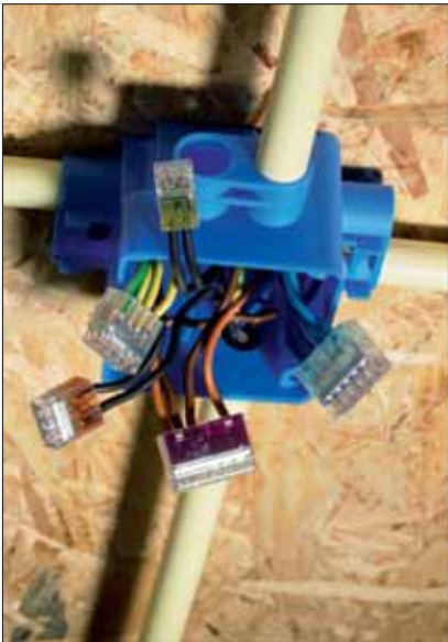
In the Netherlands, single conductors are conveniently connected with HelaCon Plus.
