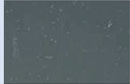
The joint has only been altered at isolated points by the UV-radiation.
