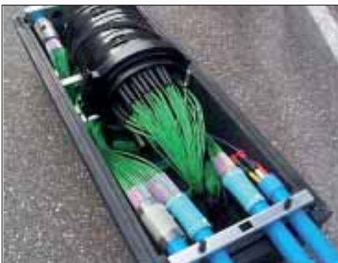
Blown cable FTTH application
