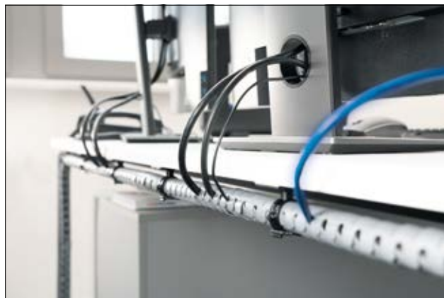
Helawrap - Office Desktop Cable Management.
