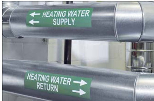
Large and highly visible pipe marking.
