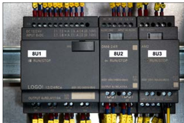
Clearly identified labels ensure easy network wire and cable management.
