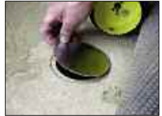
The hole is then sealed with the cavity cover plate, which fits flush with the floor surface
